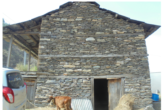
Introduction of dry stone compromising the structural integrity and Cultural authenticity.
