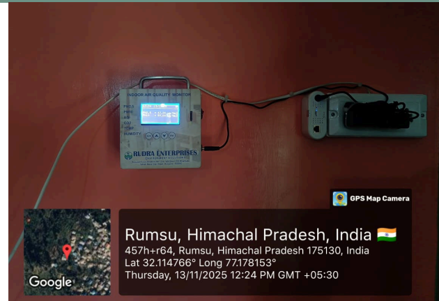
Newly installed sensors in a traditional RC building.
