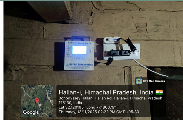
Newly installed sensors in a traditional Kath-Kunni building.
