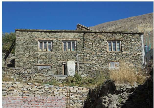
Introduction of dry stone compromising the structural integrity and Cultural authenticity.
